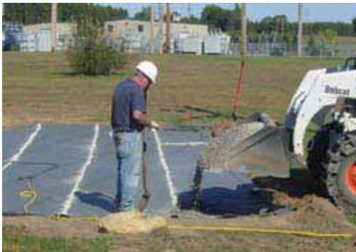
Bentonite is placed over the seams. Gravel is then placed over the material.
