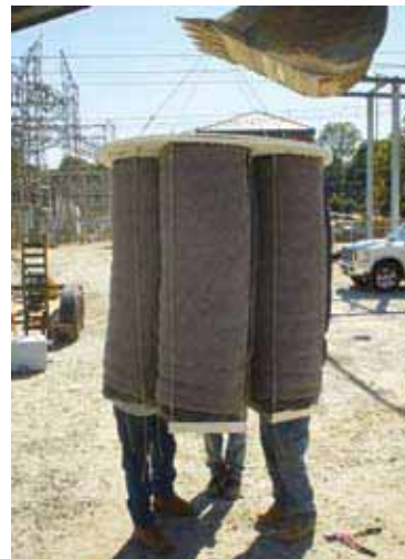
Catch basin drain filters.
