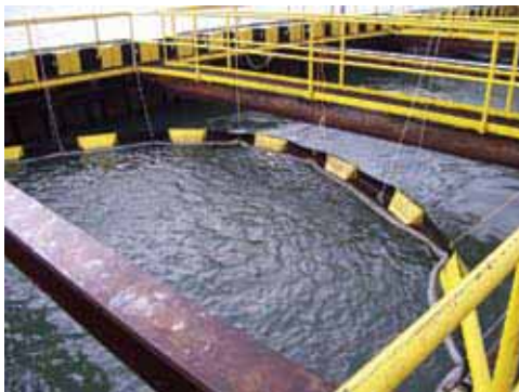
First Sheen Boom deployed in the out-fall of a major power plant.
